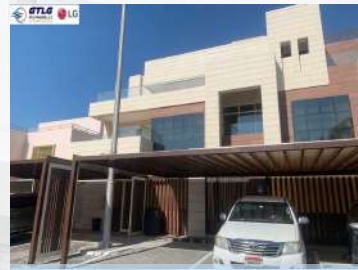
Project: PRIVATE VILLA in Abu Dhabi Description: Supply & Installation of LG Air conditioning
