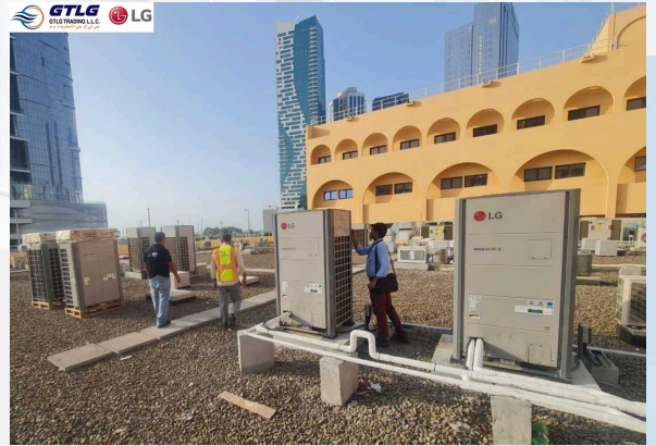
Project: CORNICHE HOSPITAL Location: Abu Dhabi Description: Supply of LG Air conditioning
