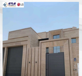
Project: PRIVATE VILLA in Abu Dhabi Description: Supply & Installation of LG Air conditioning
